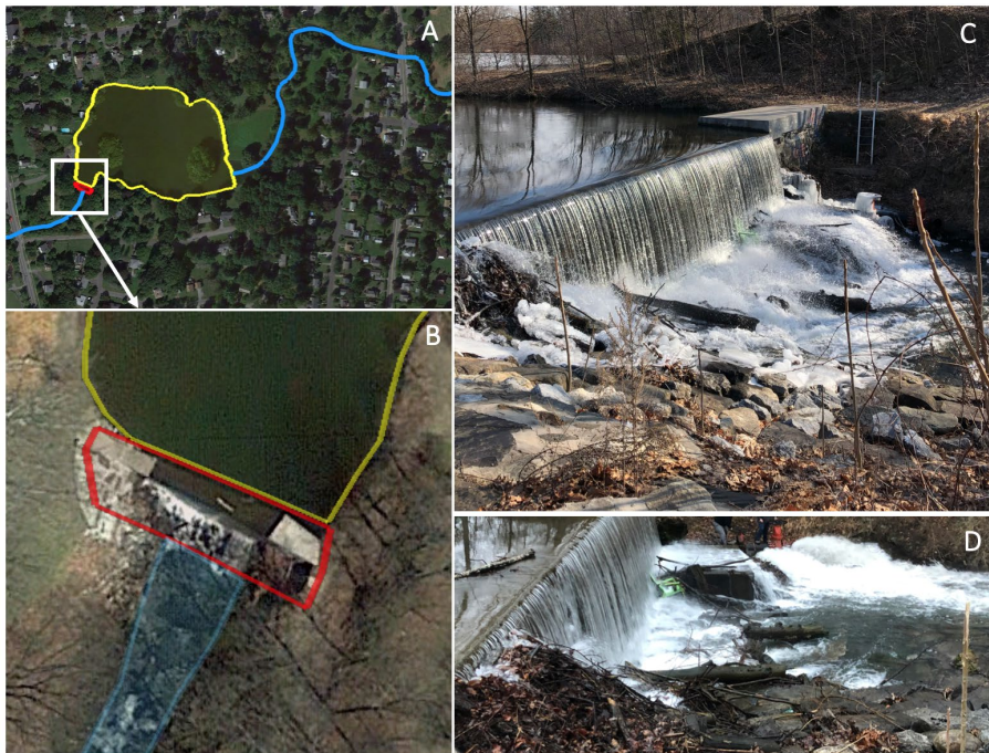
Figure 1: Overview of the Landsman Kill's flow into Crystal Lake (A), Crystal Lake, Asher Dam, and the Landsman Kill outflow outlined (B), photo taken of Asher Dam's overflow in March (C), and a photo taken of discharge of the two large valves into the outflow of the Landsman Kill in March (D).
