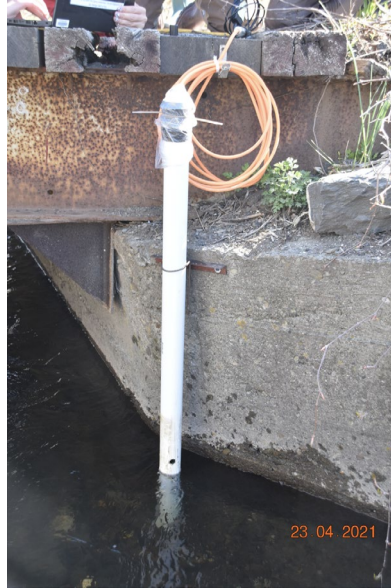
Fig. 7: Current placement of the Level Vent Logger at the Village Highway Garage
