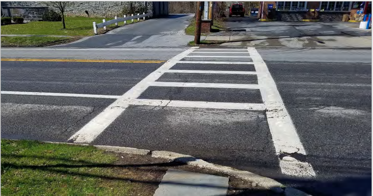
Non-accessible crosswalk at South St (lack of east side ramp and west end at gas station driveway)
