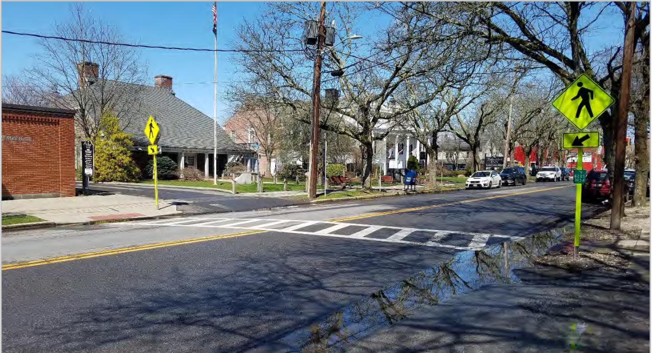
Post Office crosswalk (note ponding at both ramps)
