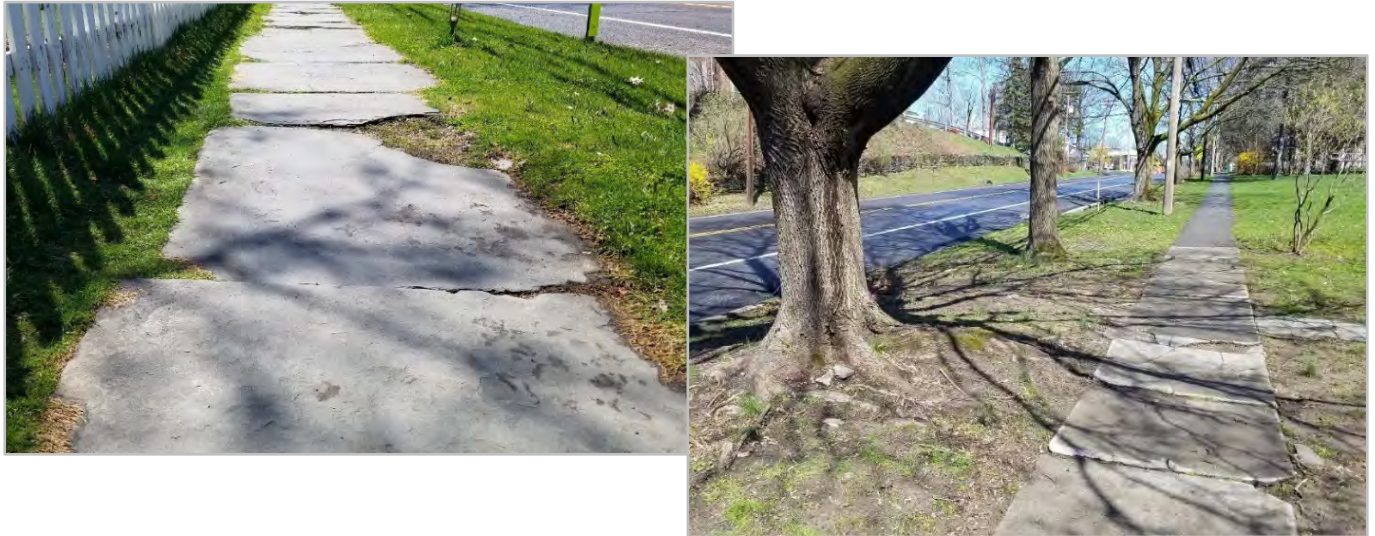
Poor condition sidewalks south of South St
