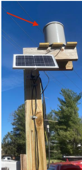
Figure 8. Installed Tipping Bucket and wiring setup.
